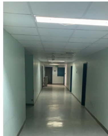
Figure 28 - Lighting System Condition in Hermel Public Hospital
