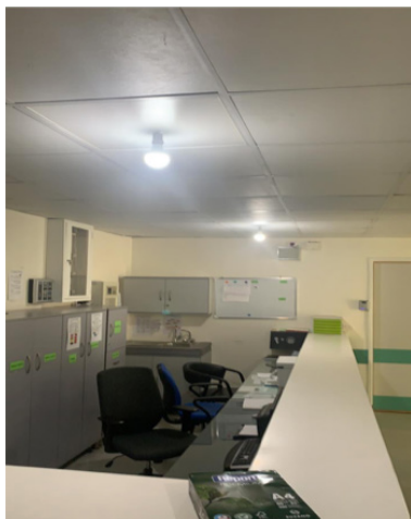
Figure 29 - Lighting System Condition in Nabatiyeh Public Hospital
